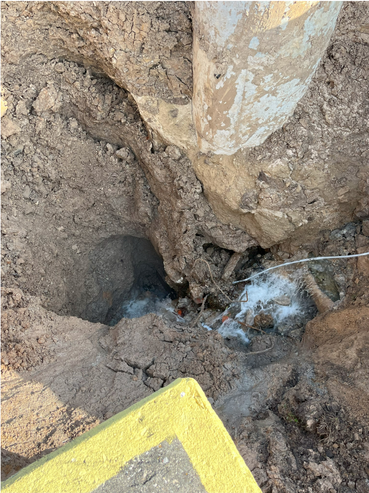
Photo of Leak. Taken January 23, 2025
